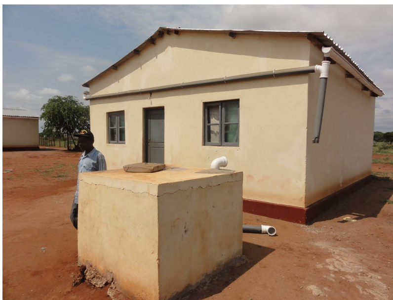
Figure 1. Type II resettlement housing with a broken water infrastructure (photo by the author, 2015).
