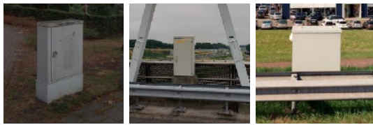
(a) CAI cabinet (b) Cabinet house (c) Cabinet house
